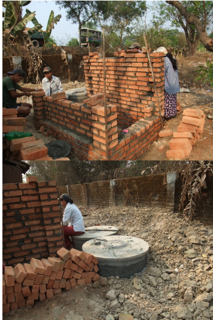
Figure 9: (Top) Myanmese workers constructing the latrine for the sanitation system. The latrine is constructed using bricks. Bricks are more robust materials than bamboo sheets that will be able to support the long vertical ventilation pipe. (Bottom) Two pits have been constructed behind the latrine to contain the wastes. A manhole is constructed for each pit for easy human access to remove the wastes when the pit is full.
