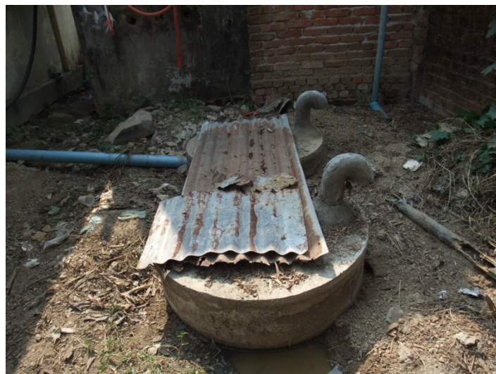
Figure 6: Two covered pits behind the toilet in a church compound in Yangon. A long blue pipe leads from the toilet carrying wastes into the pits. A curved pipe that protrudes from each of the pits is used to vent out smell. It is curved to prevent rainwater from entering the pit.
